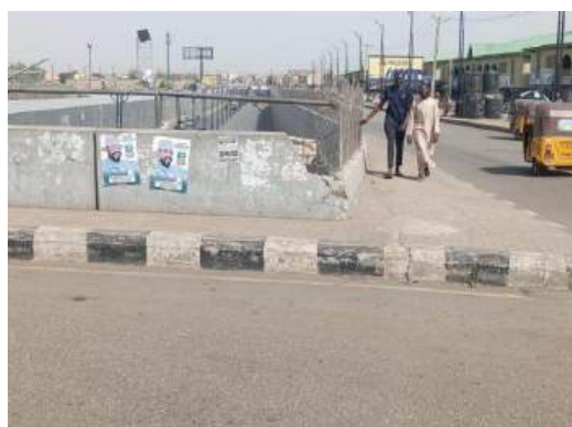
Plate 5: Structural Default along Kofar Ruwa Source: Fieldwork (2024)
