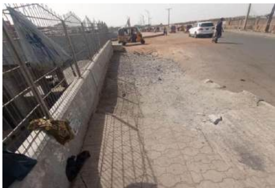
Plate 4: Structural Default along Kofar Ruwa Source: Fieldwork 2024
